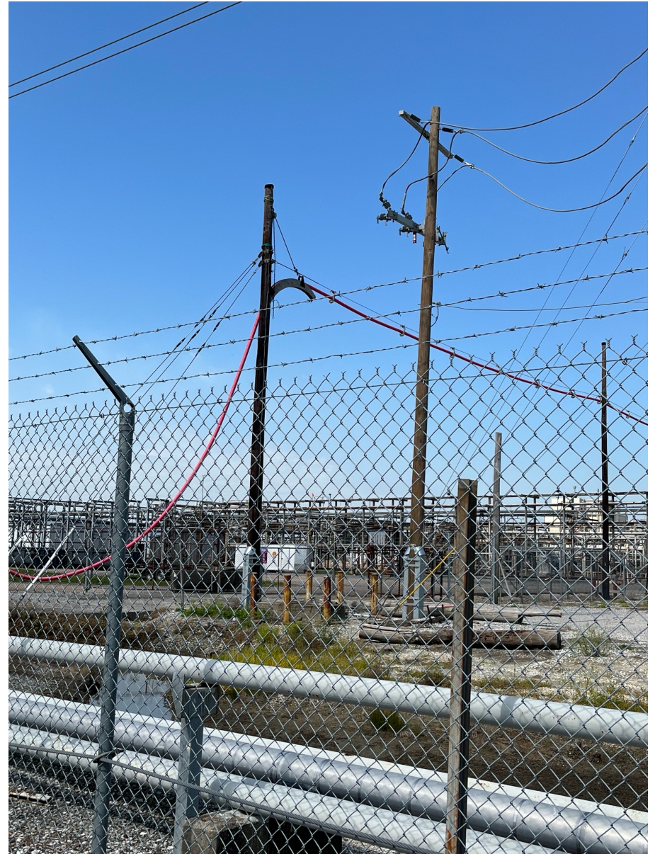
Figure 13: Pole Inside Facility, 2022
