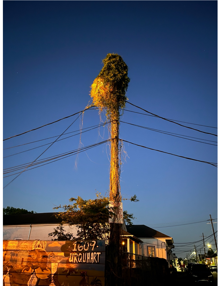
Figure 16: Pole with Growth on Top, 2023
